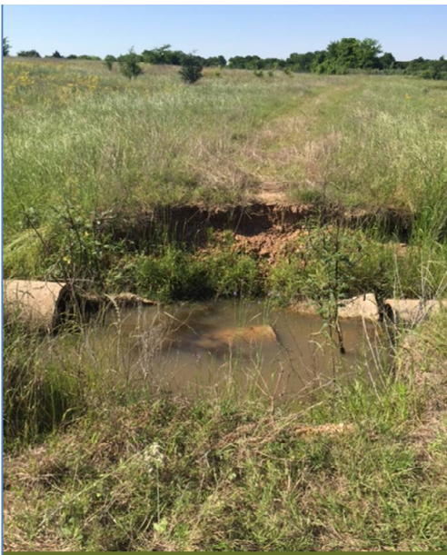
Pictured above: Bridge Washed Out by Hurrican Harvey floods.
